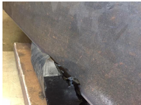
Photo 14: Here the uneven surface has put too much strain on the rubber. Since the component here was made of narrow lower plates, an upper plate should prevent the rubber from being damaged.
